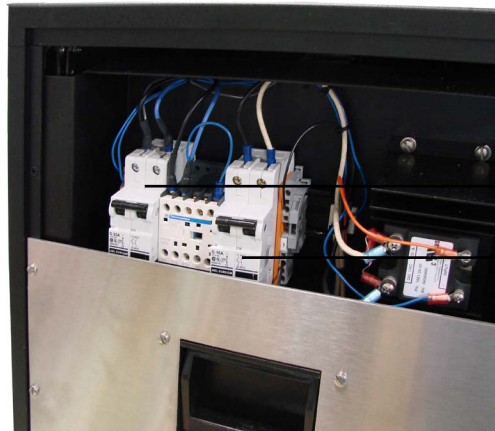
Main Circuit Breaker
